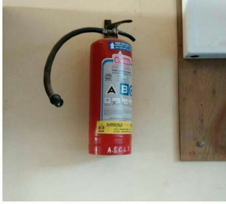
photos 13: Fire Extinguisher
